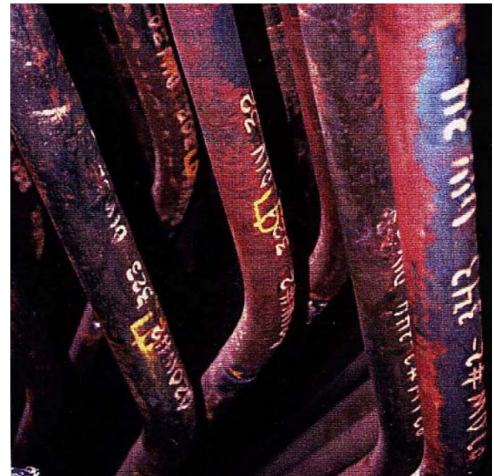
EXTERNALLY CORRODED FEEDERS AT BRUCE
