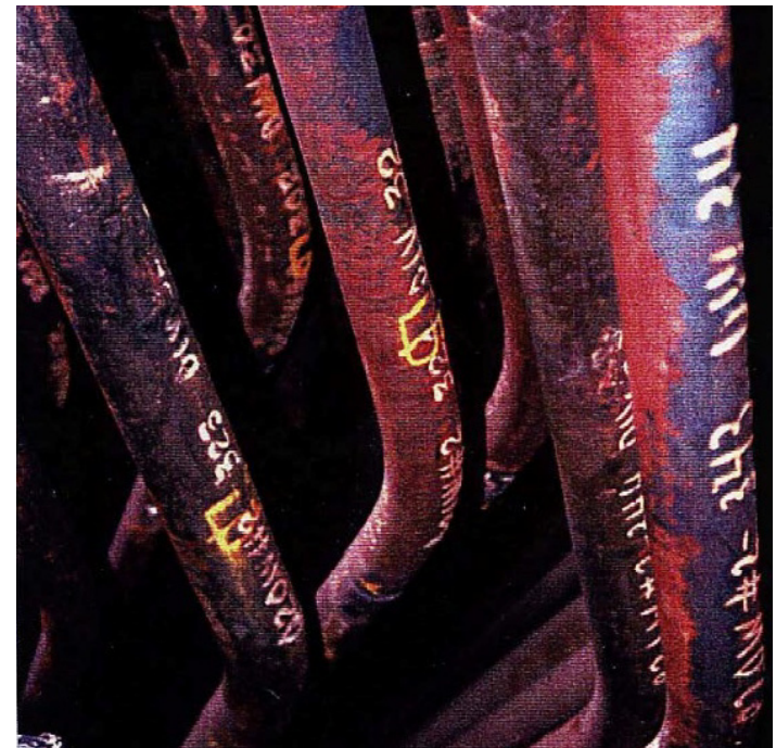
EXTERNALLY CORRODED FEEDERS AT BRUCE
